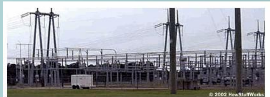
A typical substation at a power plant
