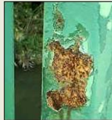
Appearance of red rust on steel, where the protective coating has failed.
