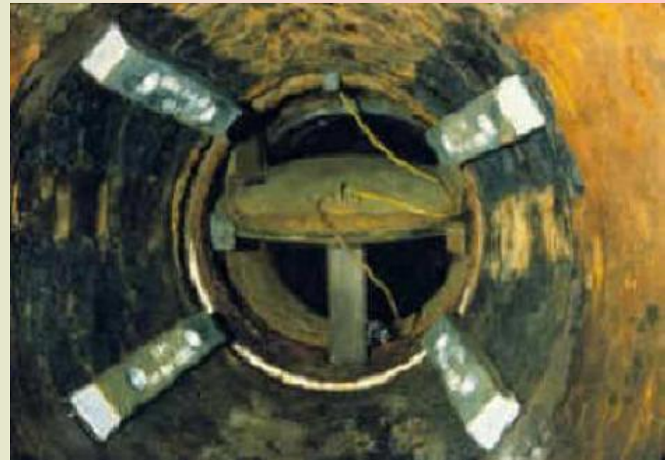
Cathodic protection with sacrificial zink anodes
